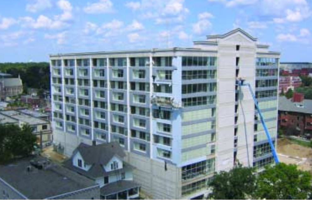
The footprint of Legacy Towers takes up about 97% of the site, making construction challenging.
