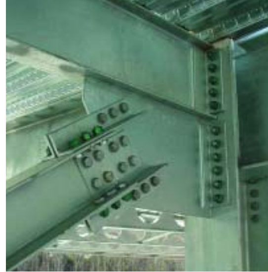
Lateral stability for the five-story parking deck was provided by chevron-braced frames. Shown above is a close-up of the connection for the lateral framing system.
