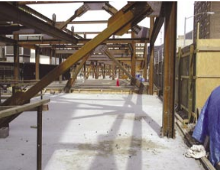
Lateral force resistance is provided by braced frames. Brace members were typically HSS shapes.
