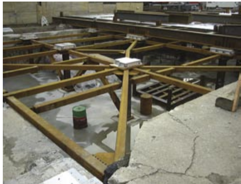
Steel transfer girders at the first floor level are supported by isolators made of springs, rubber, and Teflon.
